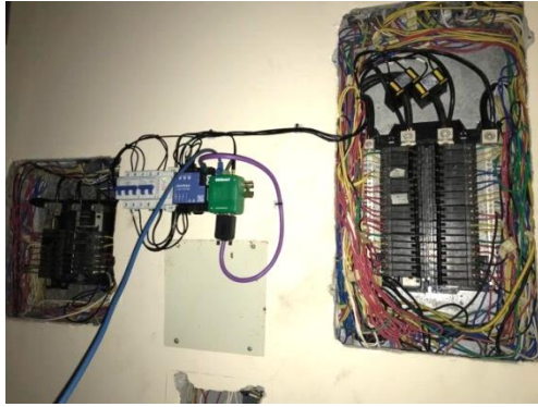
Figure 5: Energy monitoring system
