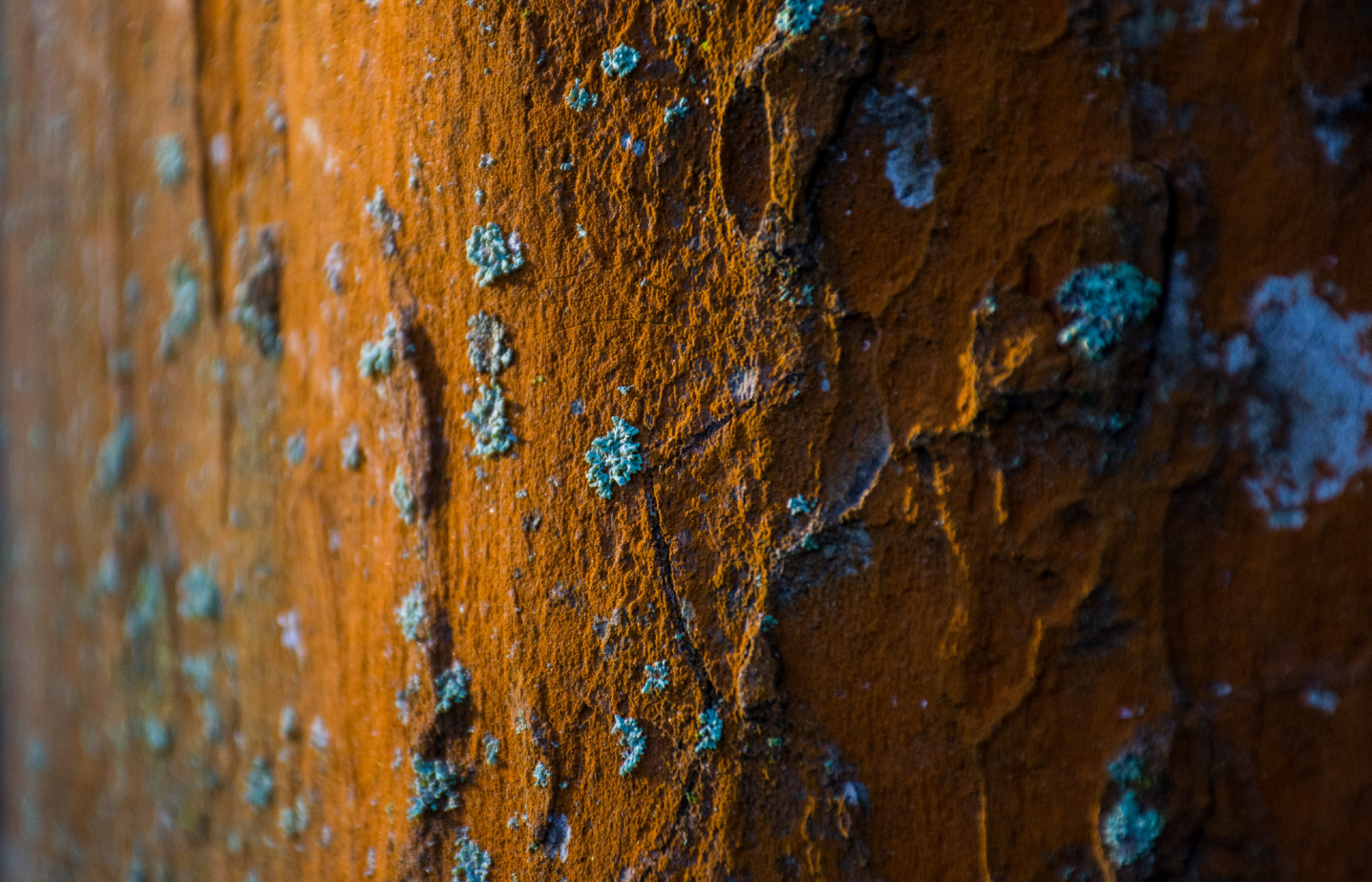
Figure 4: Corrosion in walls. Philip Ackermann. 2018. Public domain
